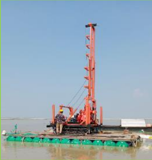
Rig Carrier Floating Stage
